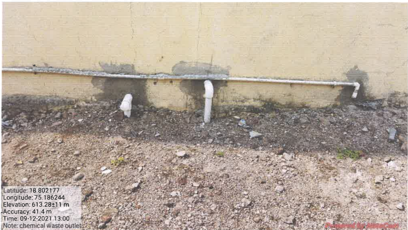
Hazardous Chemical Waste Outlet
